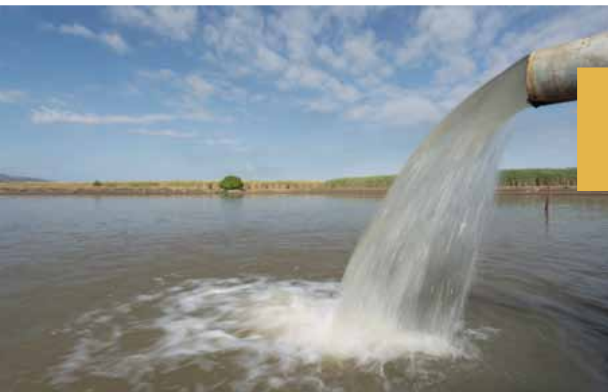
Effluent flowing into the treatment plant at Simunye mill.
