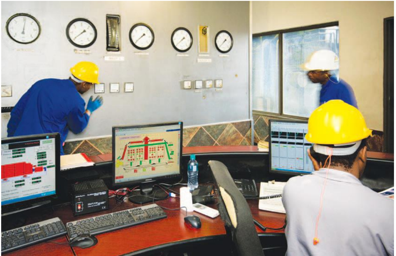
Boiler control room at the Simunye factory.
